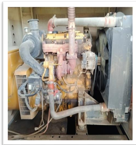
Fig. 6. Inner look of 50KVA AC Generator
