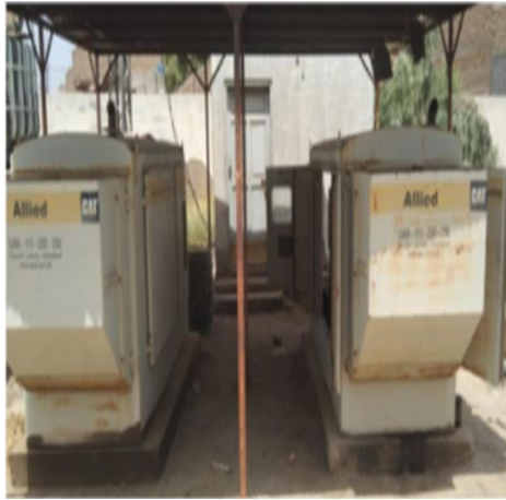
Fig. 5. Parallel Connected Generators at QUEST Campus Larkana
