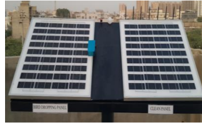
Fig 6: Initial state of the PV panels installed in the experimental setup
